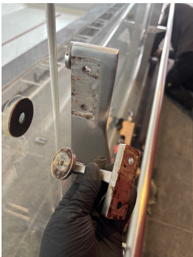
Stainless base plate - before restoration
